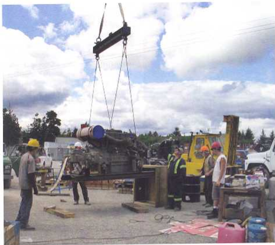
Left: Equipment is taken by truck to a disassembly suite, where it is dismantled and flown, piece by piece, to the worksite
